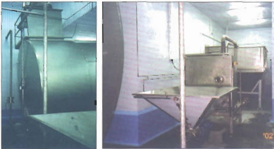
Photo 1. Daily storage tank and part of silage plant in Poland installed in 2002
